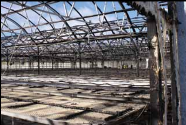
Combustible components and materials stored within the greenhouse act as fuel. It's important to identify what will be "fuel" if a greenhouse fire were to start.
