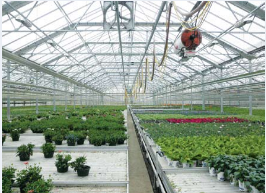
Heating systems and controls should be cleaned and checked annually.
